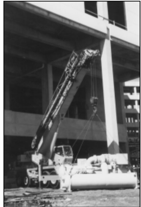
Work continues on Tampa Stadium which is set to open in September, 1998.
